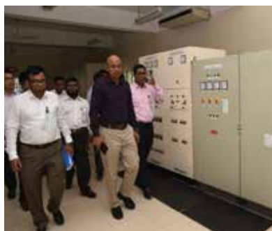
Sub-station Visit, AEPZ
