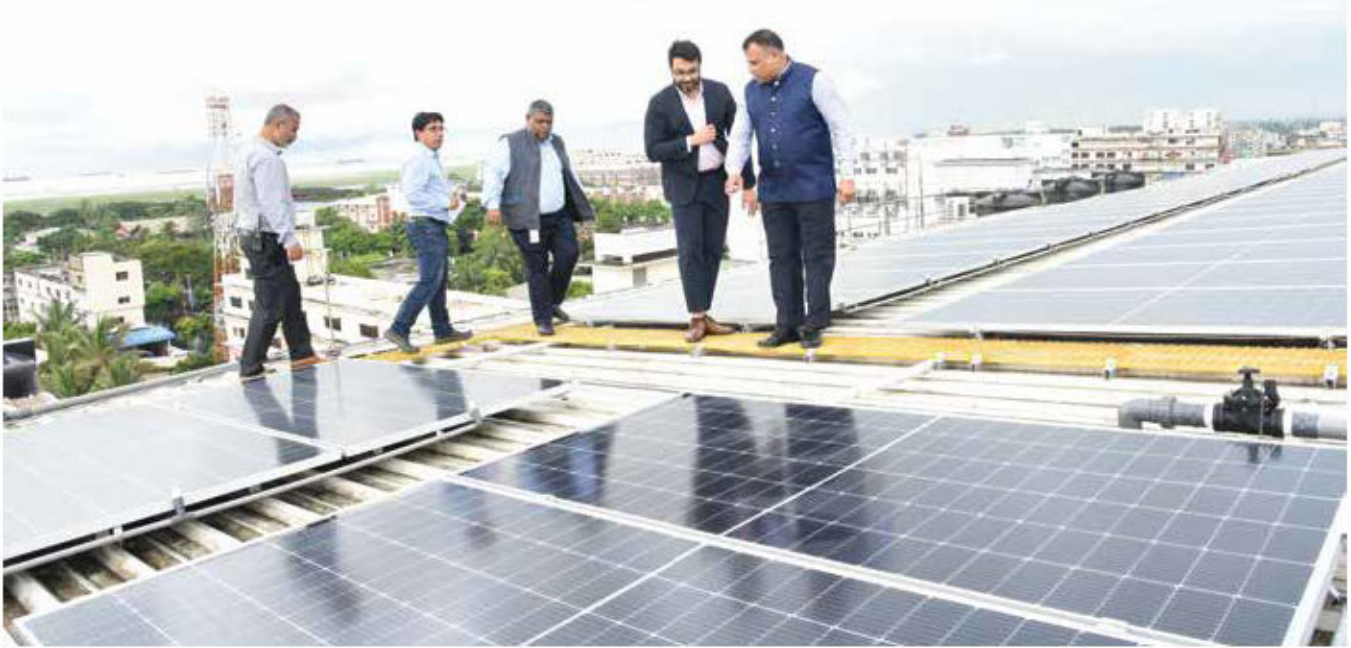
BEPZA Executive Chairman observing rooftop solar panel set up in a factory of CEPZ
