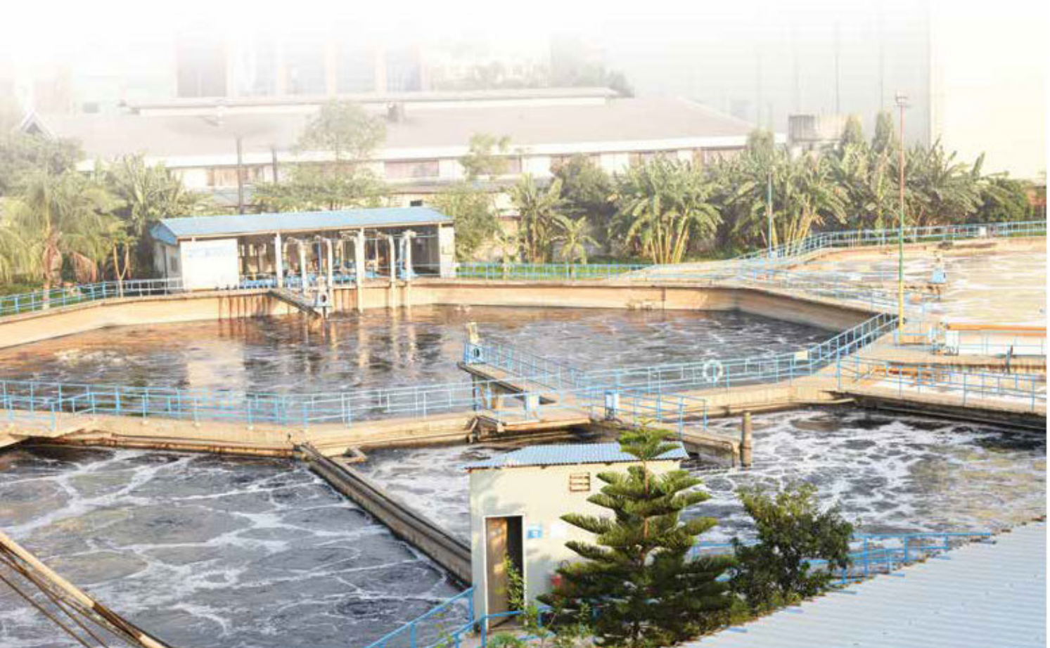
CETP of Dhaka EPZ treats the liquid waste of the factory
