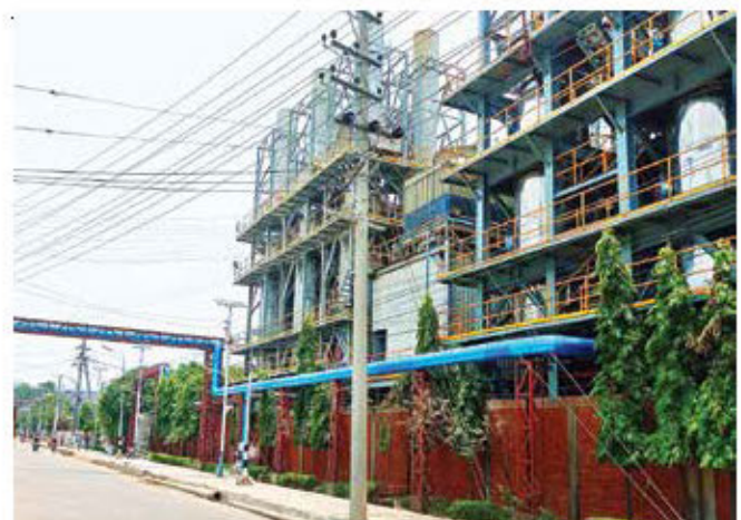
Generated steam supplies to industrial units of EPZs through pipeline
