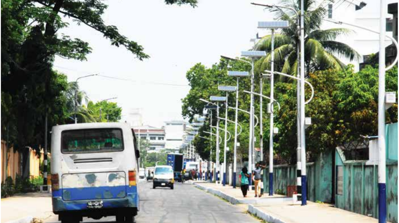
Solar Street Lights around in CEPZ area
