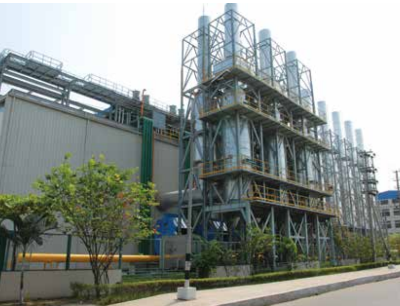
Power Plant in Chattogram EPZ
